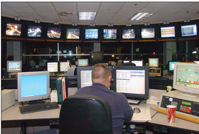
Figure 3.1—The Pennsylvania Turnpike Commission traffic control center.
