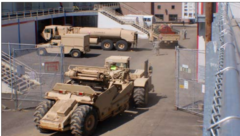
Soldiers from Forward Support Company and Headquarters and Headquarters Company, 1249th Engineer Battalion, position vehicles in preparation for work on the South Salem High school field. The soldiers are working on the field as part of their annual training.
