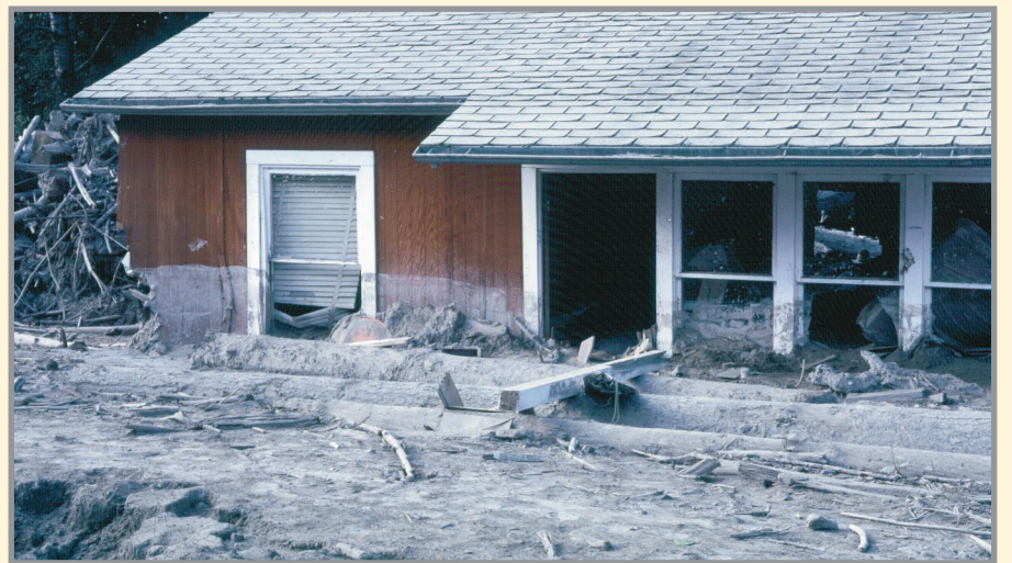
House partly buried by lahars from the 1980 eruption of Mount St. Helens. Note the high mud line on the house and large amounts of woody debris carried by the lahars. (Photo by Lyn Topinka, USGS)
