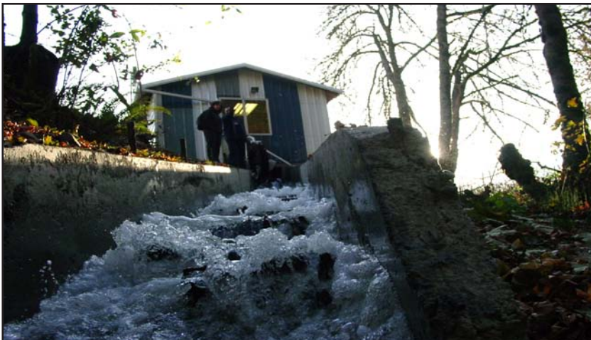
Water tumbles down into Baker Creek after it generates electricity. It is aerated before it enters the creek.
