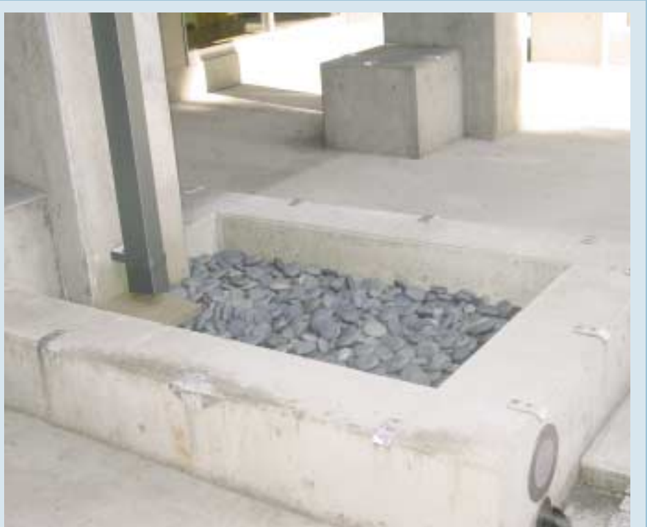
A unique water-harvesting system captures rain from the Epler Hall's impervious rooftop and pavement, and then filters it through rocks and planters to a storage tank. The water is further filtered, treated and used in the building's first-floor restroom toilets and for drip irrigation. Photo by Oregon Department of Energy.
