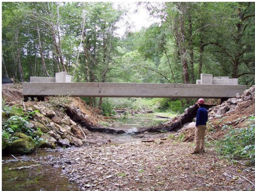
Concrete stringer bridge under construction on the West Fork Millicoma River that opened up four miles of habitat to juvenile fish migration.
