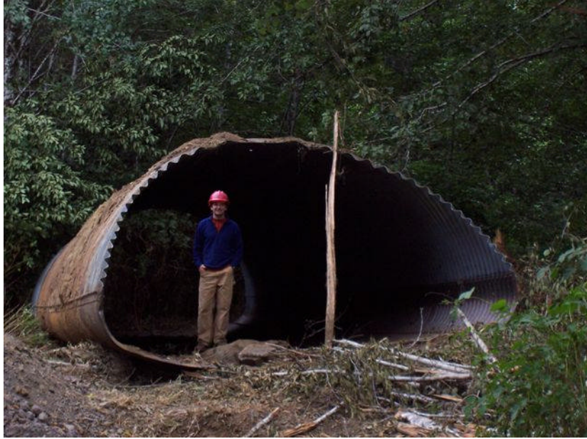
Pipe-arch removed from the West Fork Millicoma River to allow juvenile fish passage upstream and downstream.
