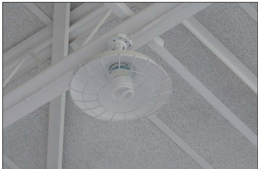
The new lights at West Hills Elementary School gym in Pendleton are much more energy efficient.
