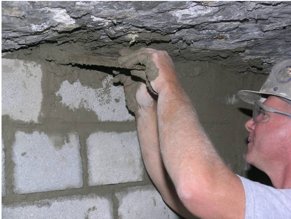
Figure B6-3.-Completely filling the gap between the top block course and the mine roof with mortar; the block were not wedged.
