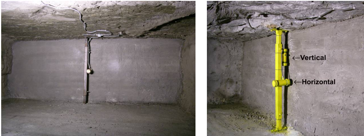
Figure 3 - Front view and side view of pressure transducers in front of seals.
