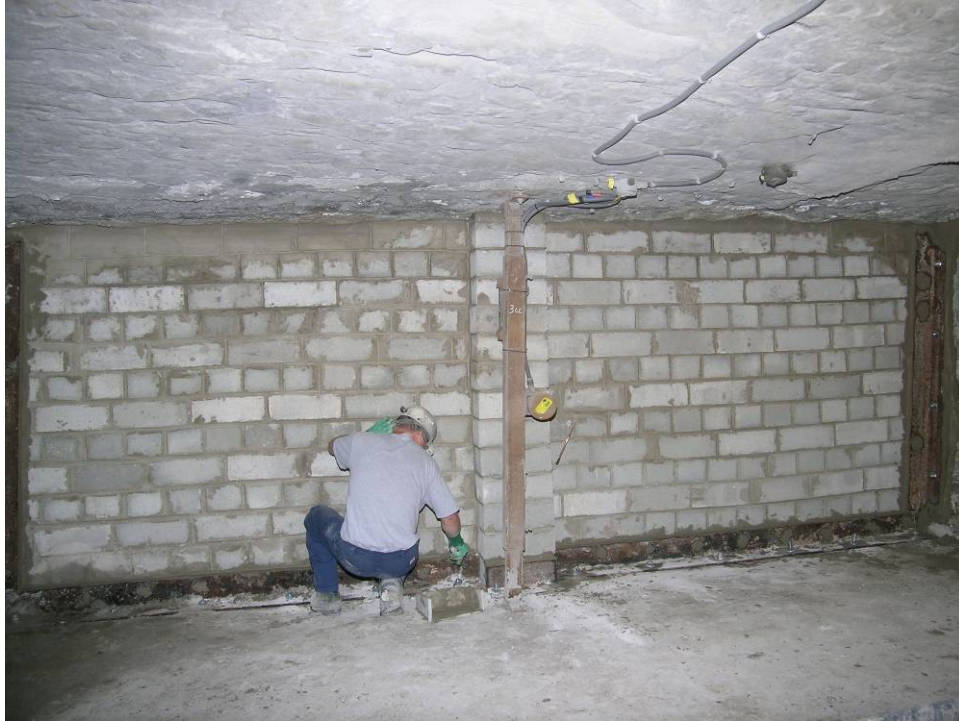
Figure B6-4.-Mortar filling any gaps that exist between the steel angle hitching and the block along the floor and ribs.
