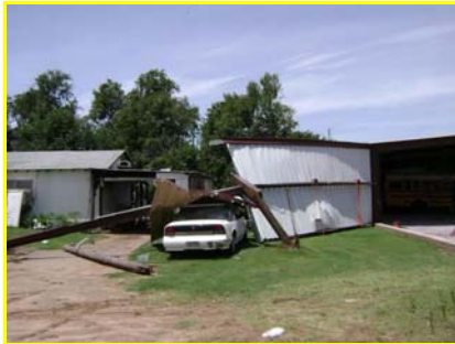
Fig. 6. Ripped frame from Wellington bus barn thrust into neighboring property.
