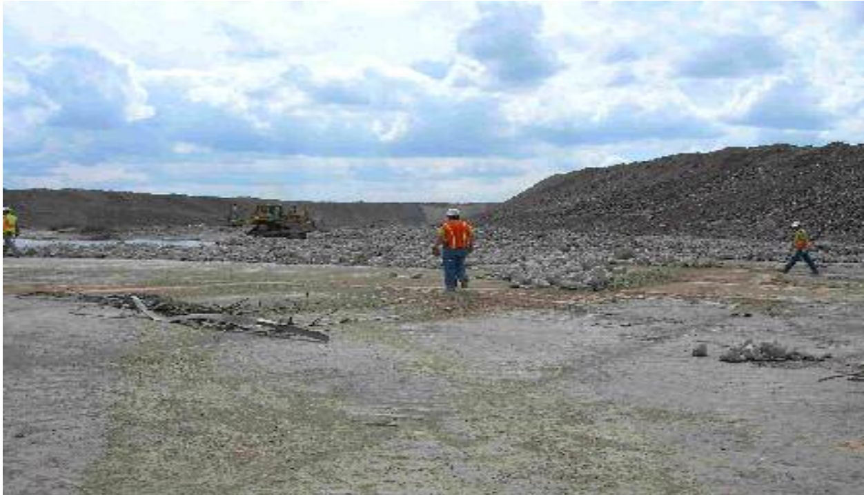
Figure 5-9. Drained upper reservoir basin showing the rockfill materials after removal of the concrete face panels. (Source: FERC Staff)
