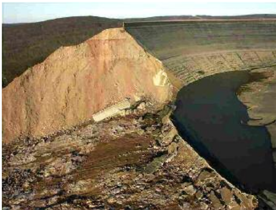
Figure 5-6. Weathered rock and discontinuous clay seam foundation just downstream of fish-pond area. (Source: FERC Staff)
