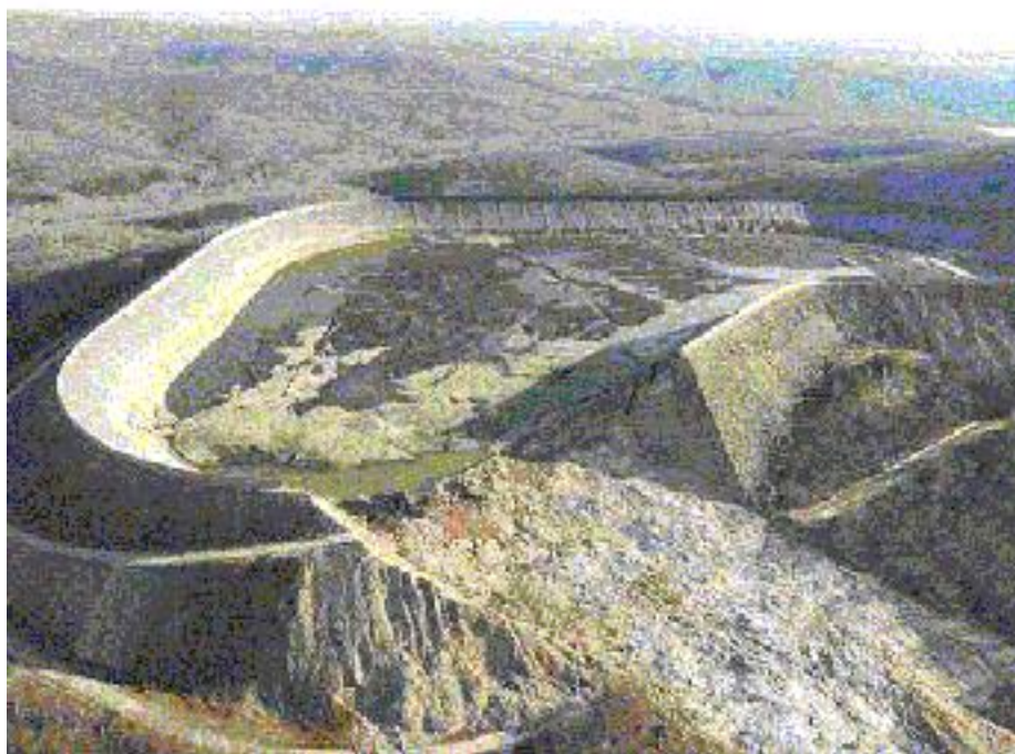
Figure 5-5. View of bedrock within, and immediately below failed embankment section. Note distribution of weathered rock (red-brown color) and topsoil (green-brown color). (Source: MDNR)
