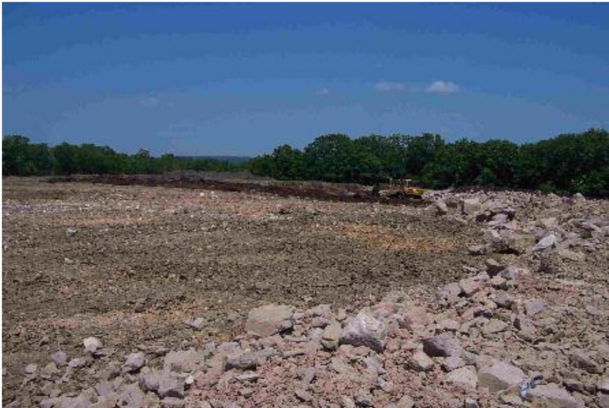
Figure 5-10. Preparation of Laydown Area 1. The fill material from the upper reservoir (sediment and concrete debris) was used to level the site. A hardfill cap will be placed over the top of the area. (Source: FERC Staff)
