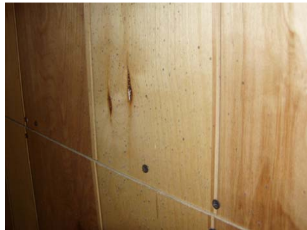
Figure 4-14b. Damage to wood panel following impingement by sparks from gerb. Lip on panel surface can be seen as line below mounting screws.
