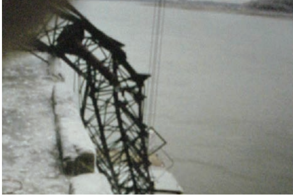
Figure 5. Boom collapse at river facility. (Photo courtesy of OSHA)
