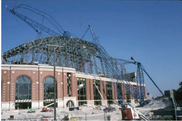
Figure 2. Heavy-lift crane after tip-over at stadium project. (Photo courtesy of John Thraen)
