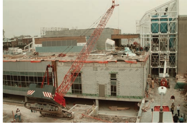
Figure 3. Crane tip-over at library expansion project. (Photo courtesy of The Blade/Toledo Ohio)
