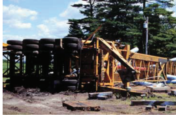
Figure 6. Mobile tower crane tip-over attempting to hoist water tank. (Photo courtesy of Iowa FACE Program)
