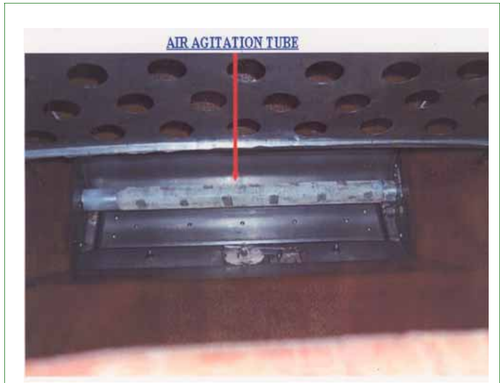
FIGURE 3-10-14 Dry Material Application System - Air Agitation Tube
