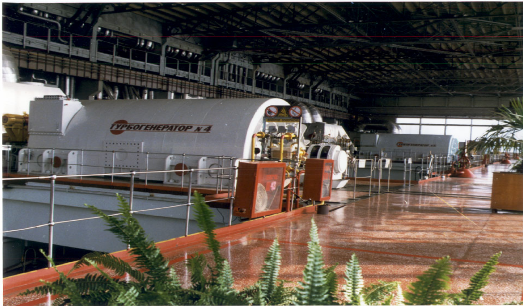
FIG. 3d. Turbine hall of the BN-600 NPP.
