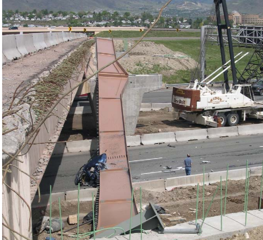
Figure 1. Fallen girder and top portion of the accident vehicle on I-70 (looking north). The C-470 bridge/overpass being widened is to the left of the fallen girder in this photograph.
