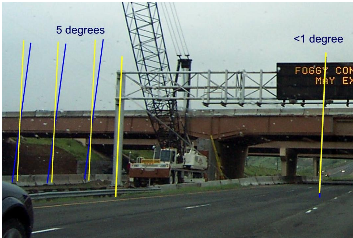
Figure 5. Portion of photograph taken by driver on May 13, 2004, while accident girder was in place over I-70. Photo has been cropped and enlarged to show area of interest; guidelines indicating vertical alignment (yellow) and estimated angle of lean of girder (blue) have been added.
