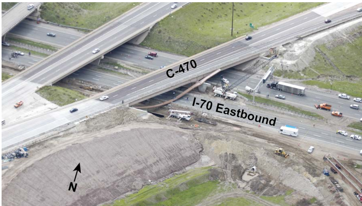
Figure 2. Overhead view of the accident scene, showing the C-470 bridge and fallen girder. (Photo source: Jefferson County Sheriff's Office)
