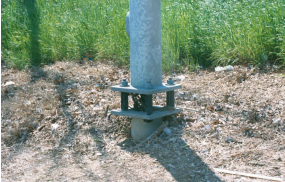
Figure 13. Exemplar light pole plate and breakaway base.
