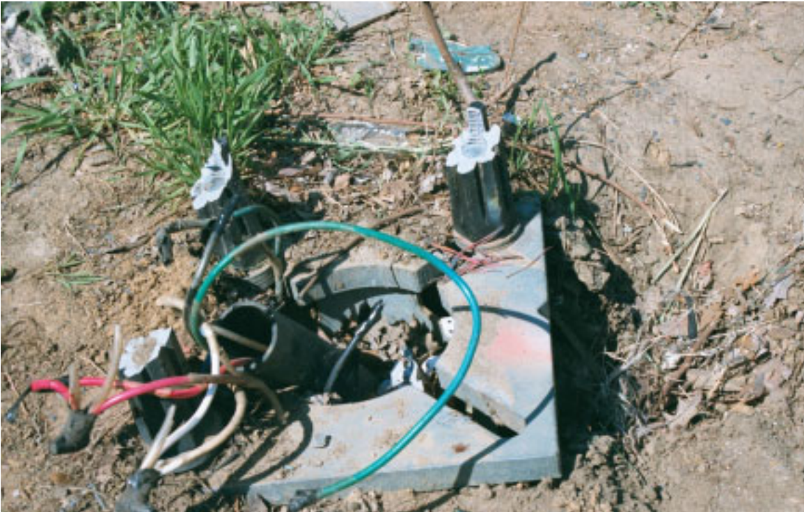
Figure 14. Light pole breakaway base mounting plate with fractured mounting nuts.
