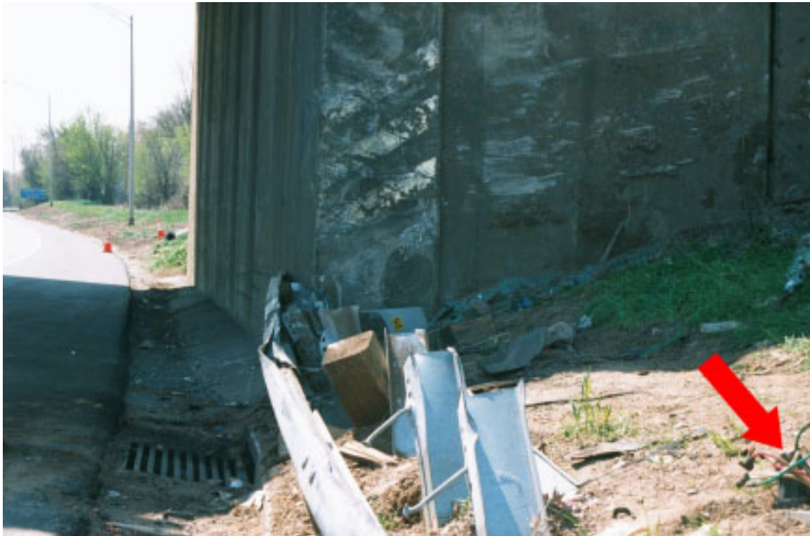
Figure 12. Guardrail damage, light pole base (indicated by arrow), and bridge abutment scrapes.
