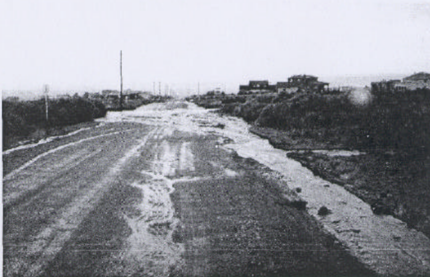
Figure 3 - Diversion caused by road crossing of arroyo
