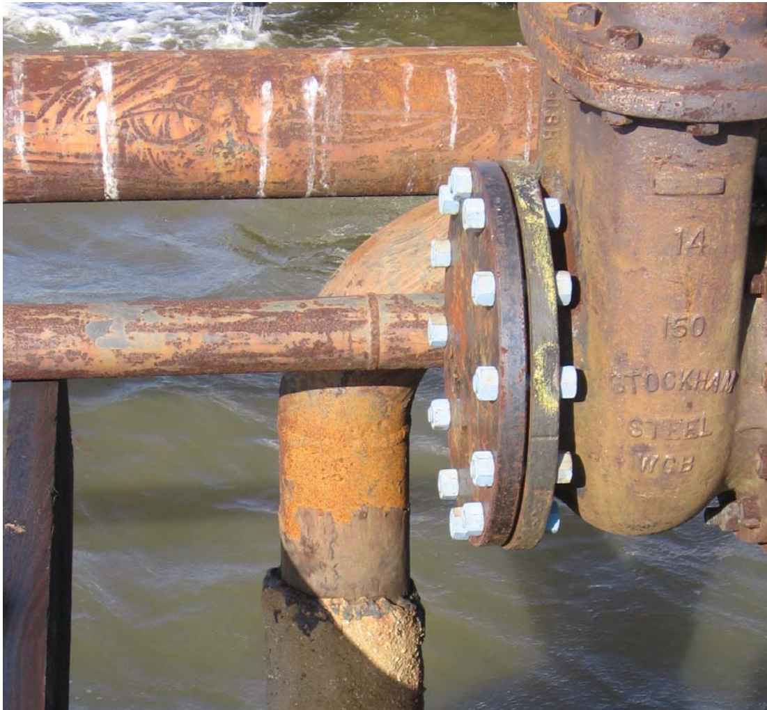
Figure 14. Beginning of the gas sales pipeline (vertical pipe entering water) at the Gulfport sales platform in the West Cote Blanche Bay oil field. The pipeline was ruptured by the Athena 106 's aft spud in an east-west section near the Gulfport platform. The pipe's concrete coating is visible above the waterline.
