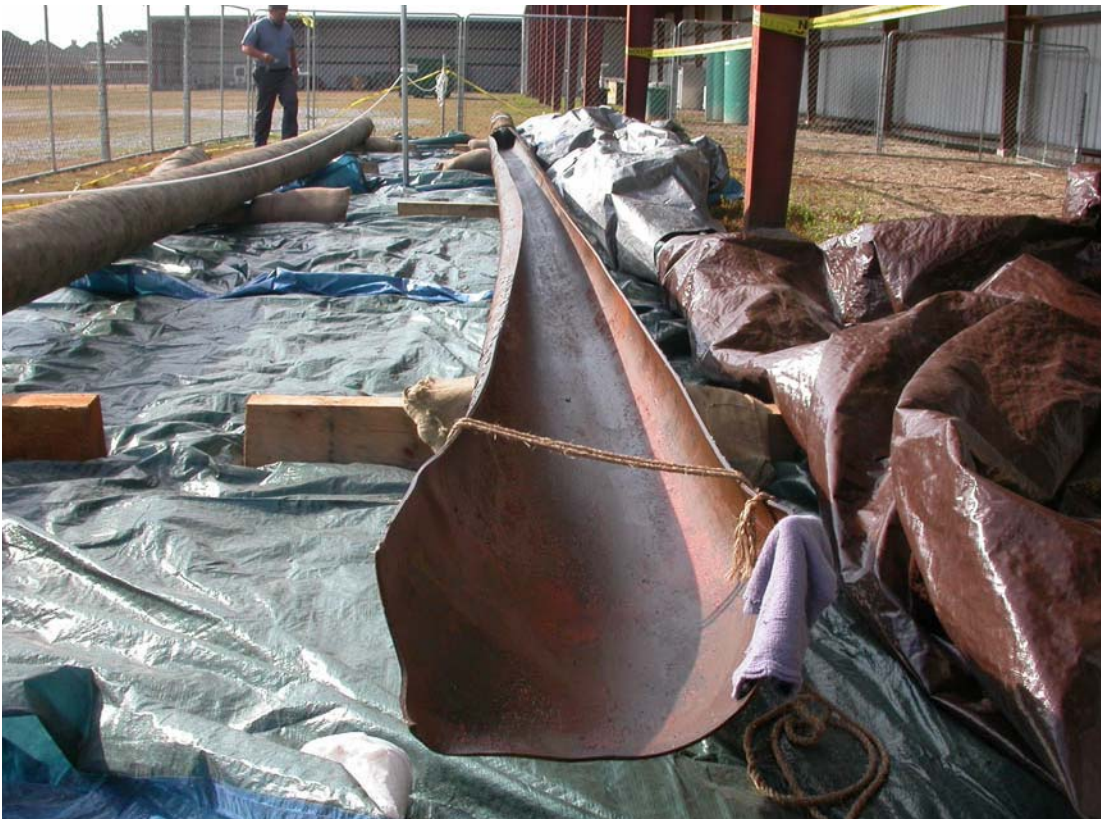
Figure 13. Fracture on the east piece of the ruptured pipeline.
