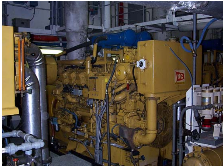
Figure 4. One of the three auxiliary diesel generators.
