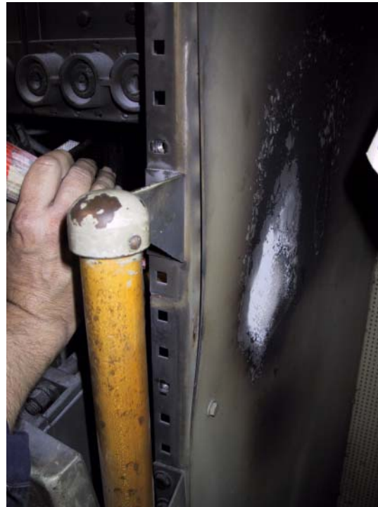
Figure 8. Closeup of heat damage to unit 12. Photograph courtesy of the U.S. Coast Guard.
