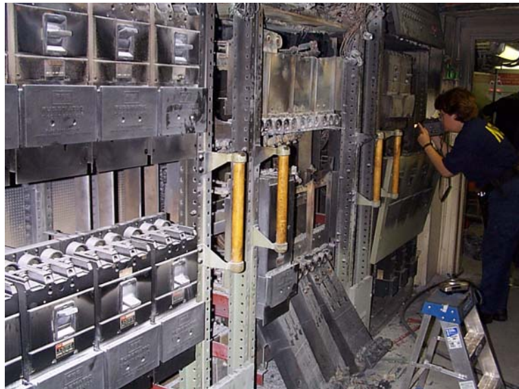
Figure 6. Units 8, 9, 10, 11, and 12 of the main switchboard. The Safety Board investigator is examining unit 12.
