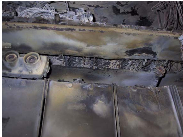
Figure 10. Closeup of hole in steel plate in unit 10. Photograph courtesy of the U.S. Coast Guard.
