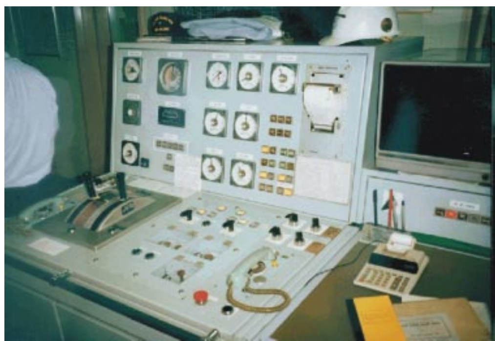
Figure 4 -- Engineering control, monitor, and alarm console
