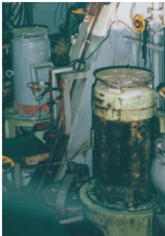
Figure 10 -- Bright Field No. 1 (left) and No. 2 lubricating oil pumps
