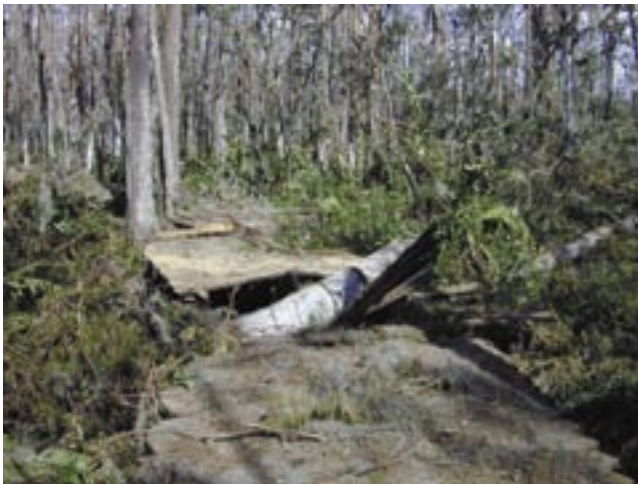
Walkway and supports severely damaged on the Cypress Swamp Boardwalk
