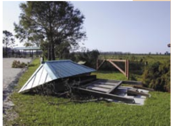
Destroyed Everglades Trail kiosk at the beginning of the Marsh Trail
