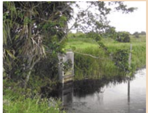
Figure 1. Part of the new riser and culvert system designed to manage water inputs and outputs of the east compartments.
