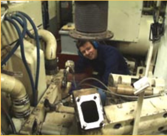
Assistant Engineer Aaron Streitberger "wrenches" on the main engine deep within Discovery Bay's noisy engine room.
