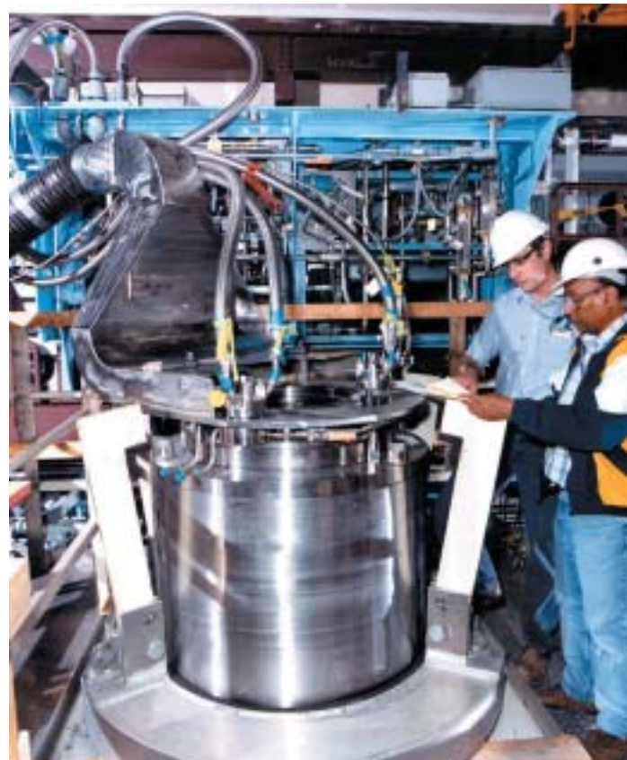
Spent fuel in multi-canister overpack being dried at Cold Vacuum Drying Facility
