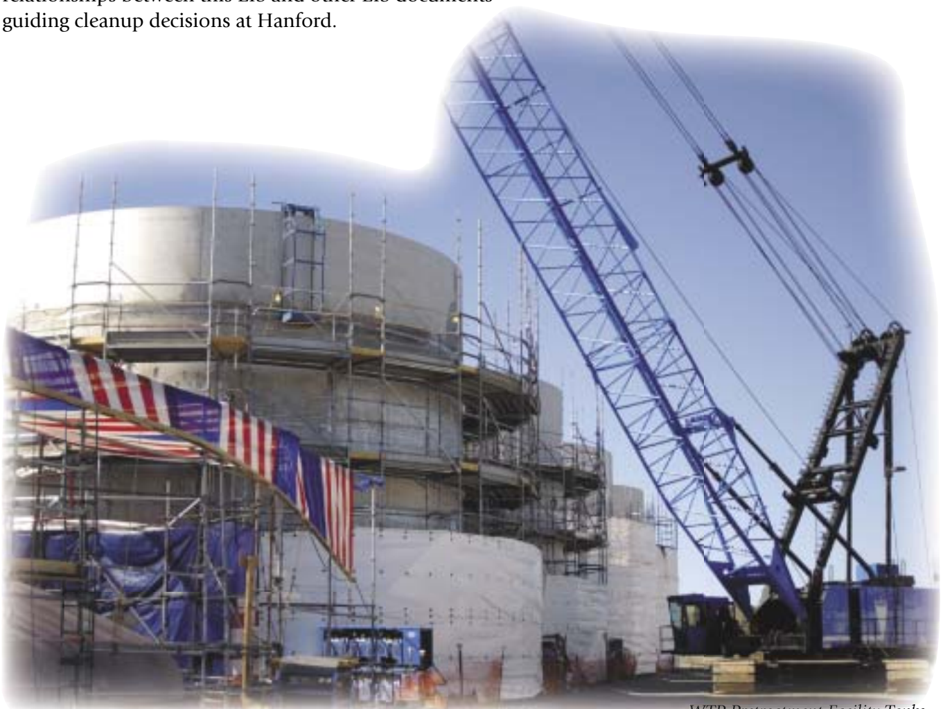
WTP Pretreatment Facility Tanks
