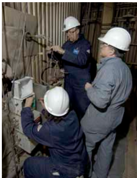
NETL researchers Sophie Bullard, Bernie Covino, and Steve Matthes (left to right) install a new corrosion sensor during the 5-month field trial.
