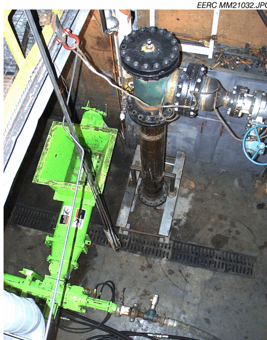
Figure 13. Pump system configured for pumping sludge into pressurized vessel – top view.
