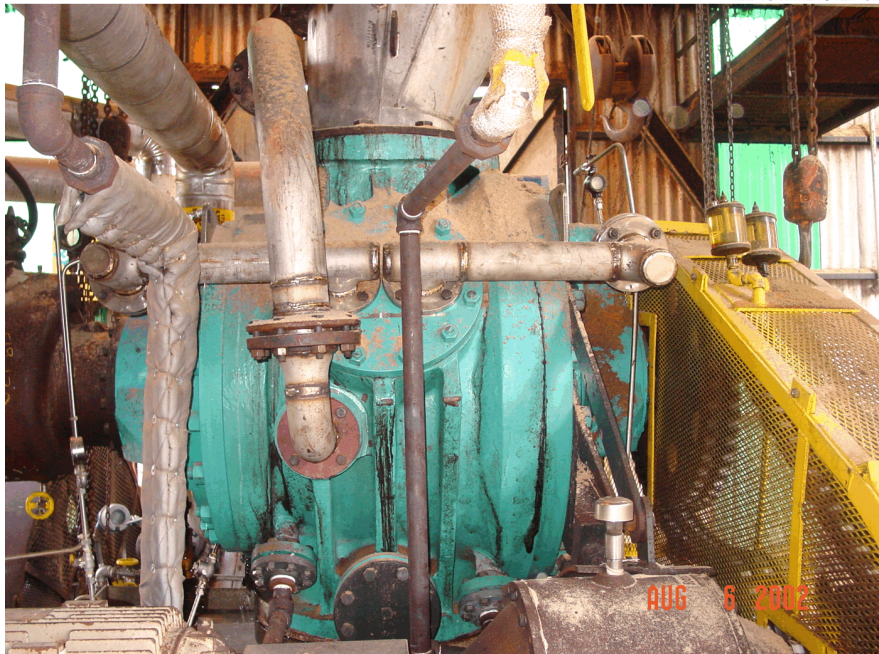
Figure 41. Rotary feeder used in sawdust pulping process – side view.
