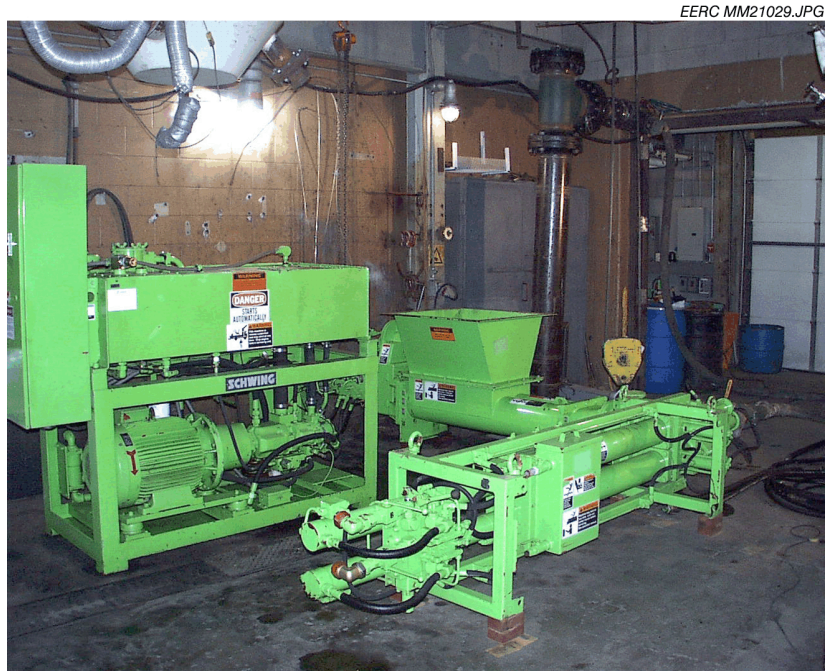
Figure 10. High-solids sludge pump, twin-screw feeder, and power pack used at the EERC.
