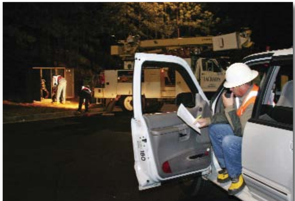
Night call: a Jackson Electric Membership Corp. crew makes a nighttime repair to keep the lights on for some of its members. The co-op recently received a $166-million loan from USDA Rural Development to provide 2,100 miles of new lines and make system improvements. Photo courtesy Jackson Electric
