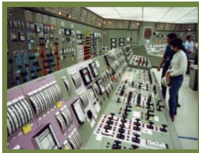
Nuclear power plant control room.
