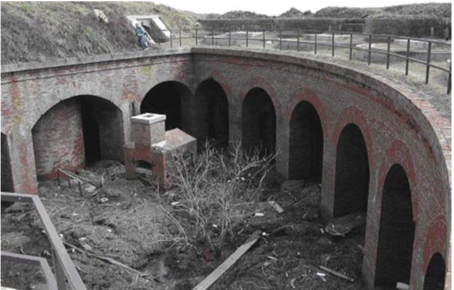
Battered by Hurricane Katrina, the masonry fortification of Fort Massachusetts was one of numerous Gulf Coast sites that experienced serious storm damage. Constructed in 1859 to provide military protection for New Orleans and the Gulf Coast, Fort Massachusetts is now part of Gulf Islands National Seashore. NPS PHOTO
