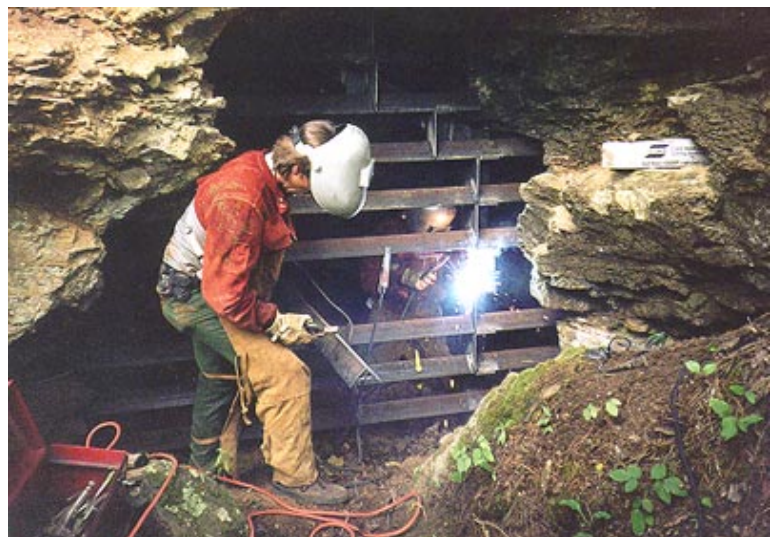
Installation of steel gates at underground mine openings in the Rush mining district of Buffalo National River conserve critical bat habitat and eliminate unsafe visitor conditions.
