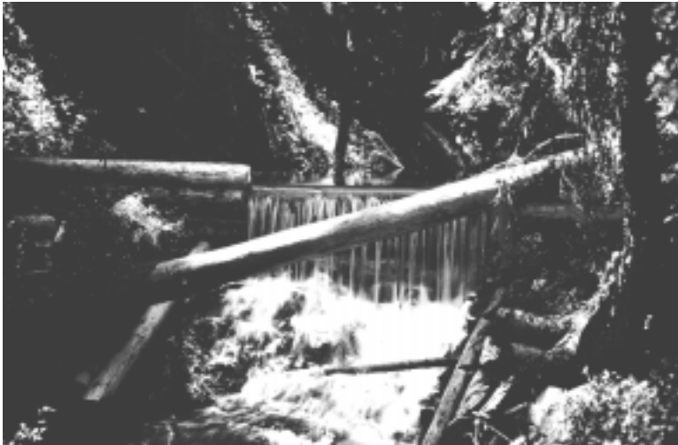
At Crater Lake National Park log and rock immigration barriers were constructed to prevent upstream re-invasion of non-native fish.
