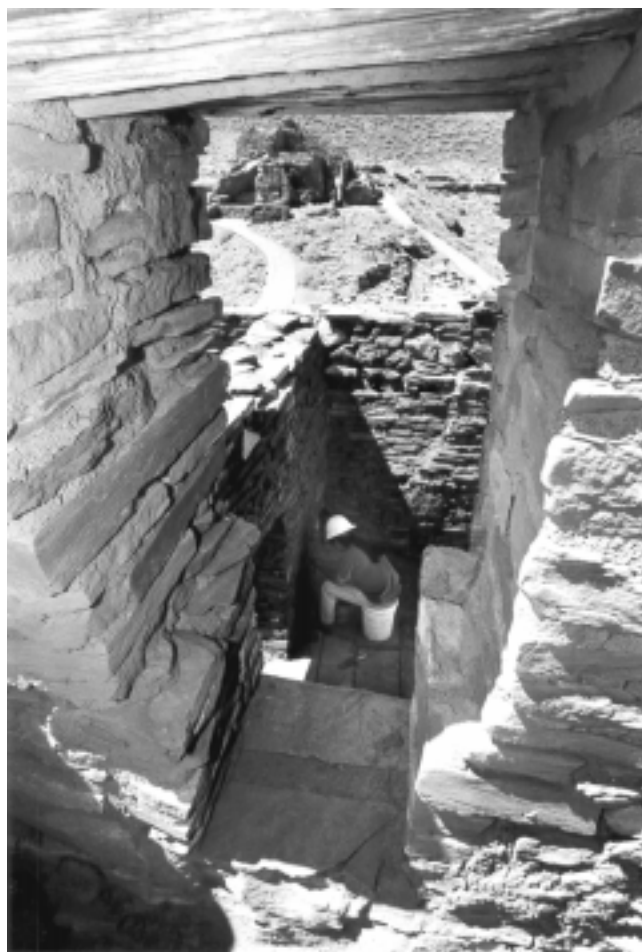
NPS stabilization workers repaired an interior room of Arizona's Wupatki National Monument as part of the NPS Vanishing Treasures Initiative.
