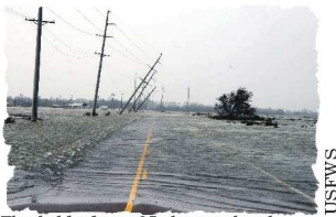
Flooded highway 27, damaged and downed power lines outside of Hackberry, LA, on the way to Sabine NWR
