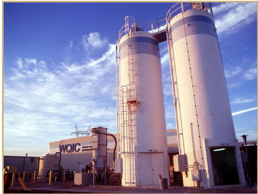
Water Quality Improvement Center in Yuma, Arizona.
