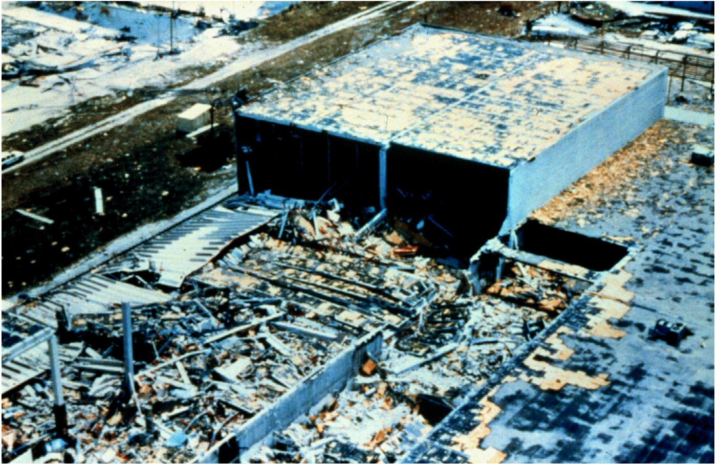
Levitz furniture warehouse, west of Whispering Pines, Florida, shows extensive wind damage.
