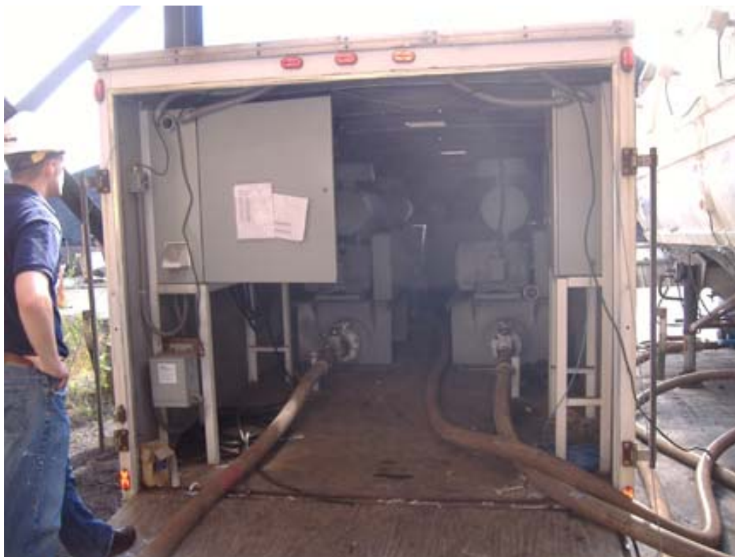
Figure 2. Trona Injection Trailer Blowers and Controls.
