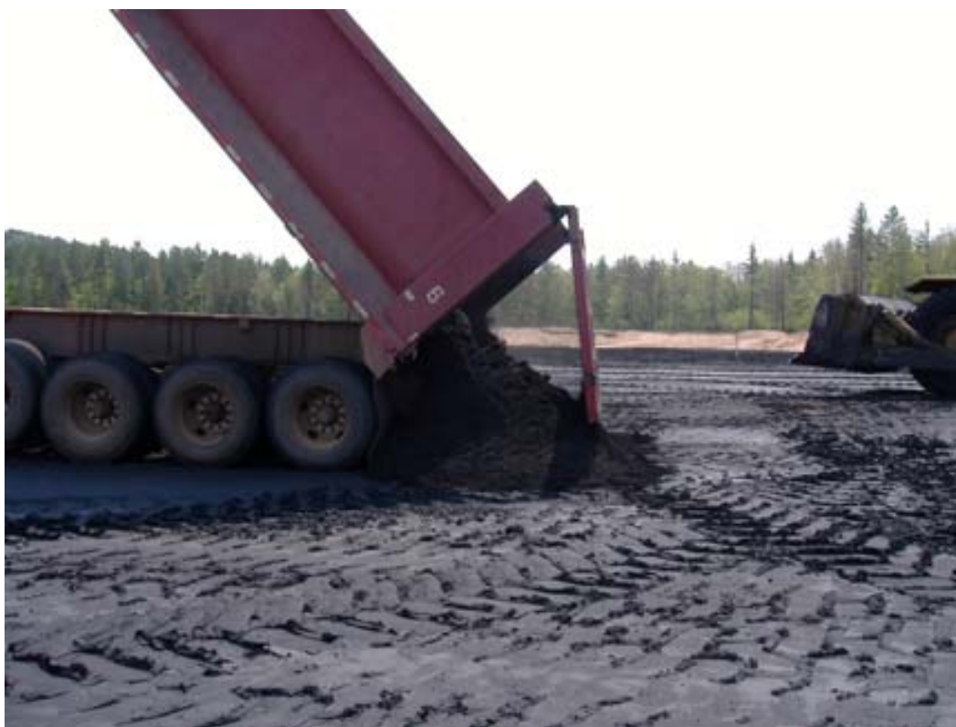
Figure 5. Unloading Reacted Trona/PAC/Ash Mixture
