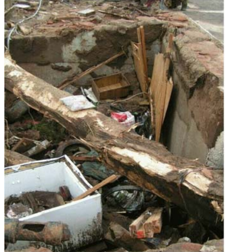
Basement filled with debris. The couple were along the west wall which is to the right.
