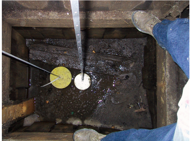
Figure 9. Stilling well at Suwannee River near Wilcox on January 4, 2002. (Photograph by Stewart Tomlinson, USGS, Tallahassee, Florida.)
