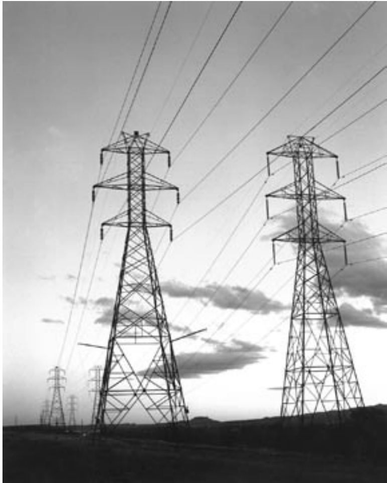
Transmission lines. Photo courtesy of Department of Energy.
