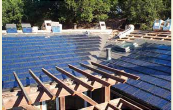
Roof mounted photovoltaic can supply household energy needs.
