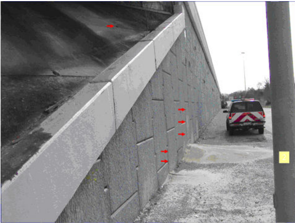
Examples of MSE retaining walls exhibiting loss of select backfill
