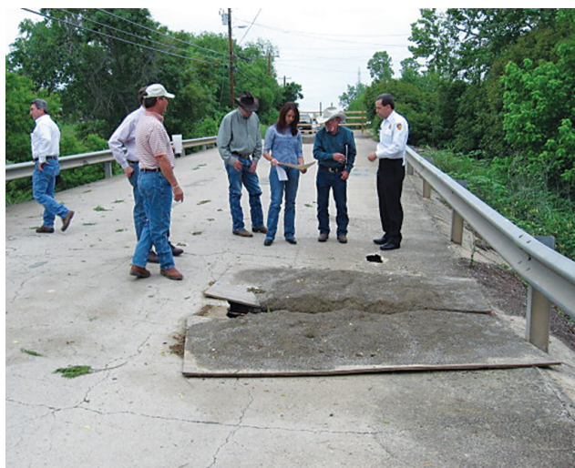
Representatives from NRCS and the City of Marble Falls examine damages to the bridge on Pecan Valley Drive in Marble Falls. Photo by Margaret Hardin, Langford Community Management Services.
