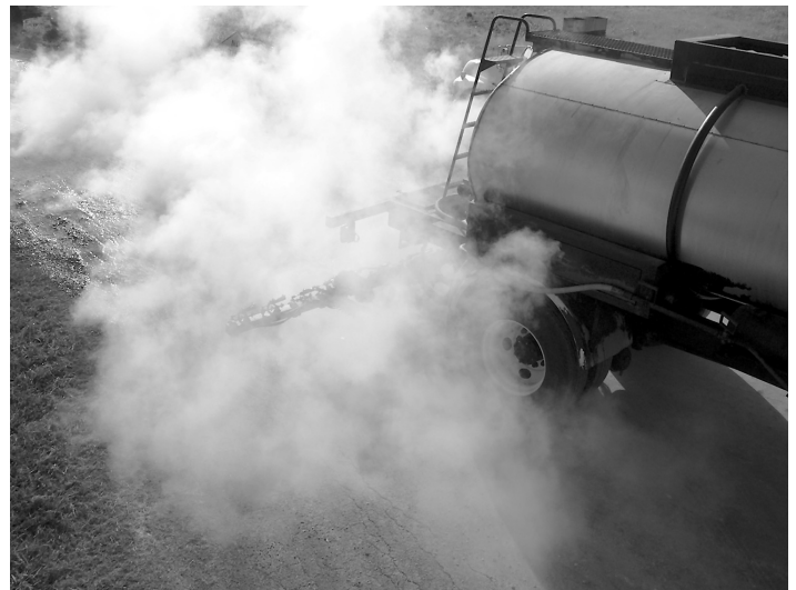
Smoke rises as TXI applies hot oil over a road in Ellis County, Texas. The resurfacing of the road was part of a field test for a new TXI product developed to use recycled materials and increase the strength of the roadbed.
