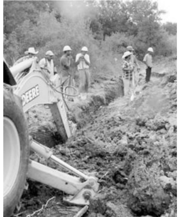
Residents of Kennedy Ridge initiated the effort to bring water and wastewater services to their community. They also provided the labor to install 14,600 linear feet of pipeline.
