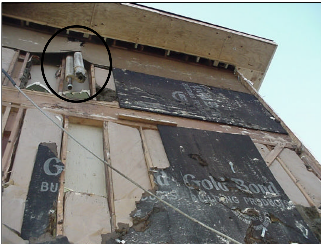
Figure Twelve. HVAC pipes on north end of Section 3.
