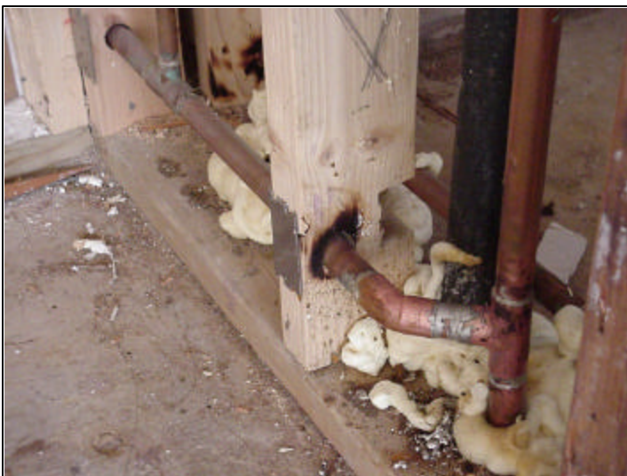
Figure Five. Charred wood observed in adjacent building undergoing renovation.
