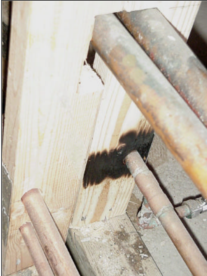
Figure Four. Charred wood observed in adjacent building undergoing renovation.
