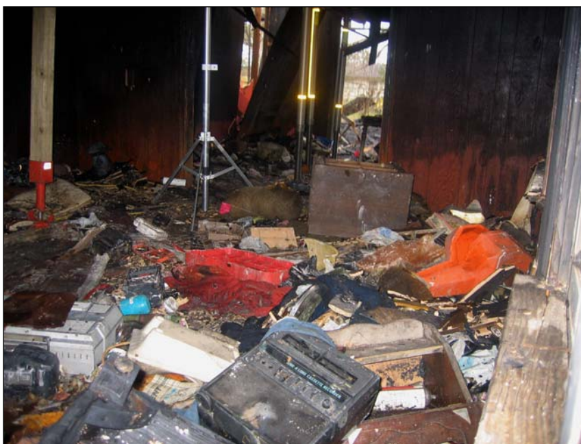
Interior of 8510 Brandon (post fire)
