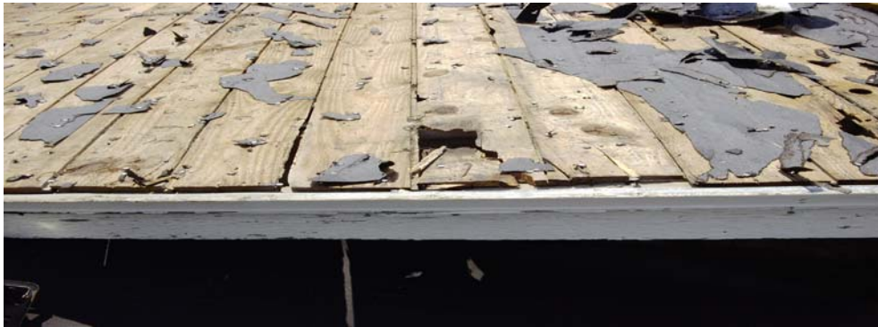
Older Deteriorated and Damaged Deck (Board Decking)
