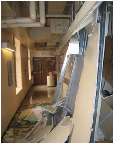
Figure 2 - Hallway Outside Laboratory Showing Explosion Damage
