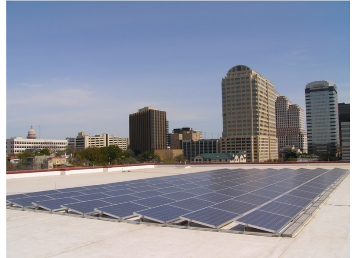
23.3 kW, ABC Bank, Austin, TX
