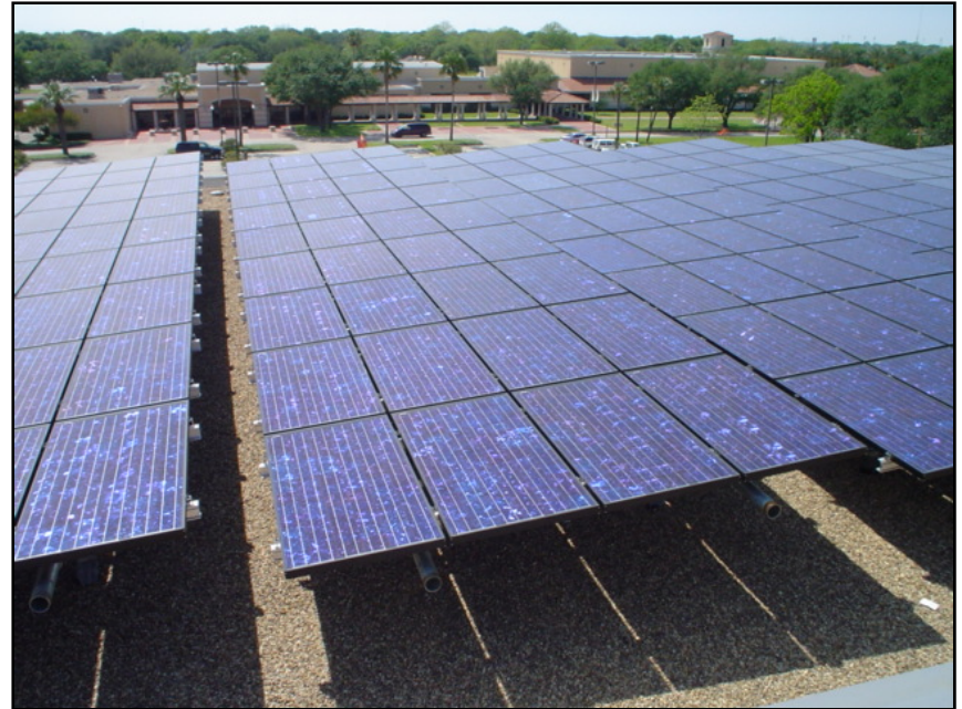
50.1 kW, Lowry Fitness Center, Texas City, TX
