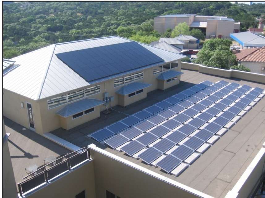
23 kW, The Overlook at Rob Roy, Austin, TX
