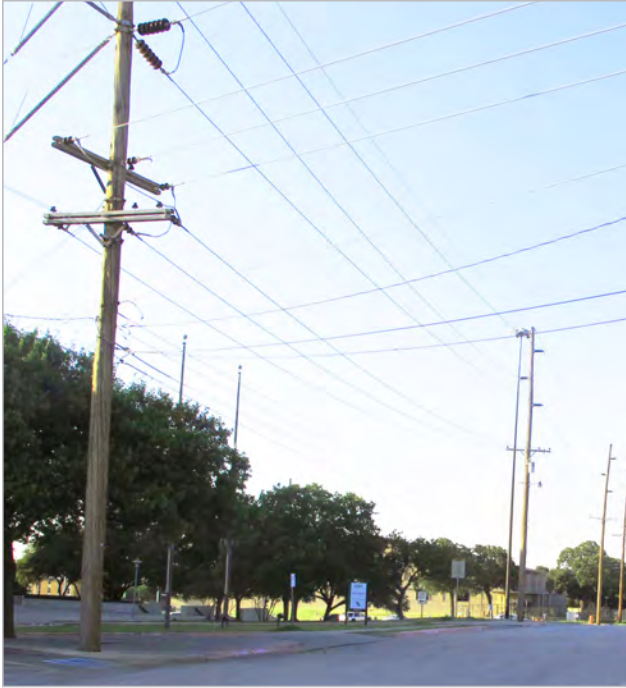
Existing Maple Street electrical transmission poles
