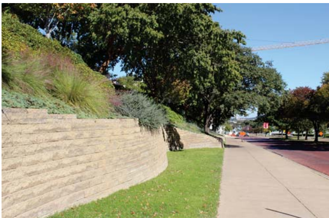
Retaining Walls Exist at Multiple Places on Campus to Hold Back Earth Elements
