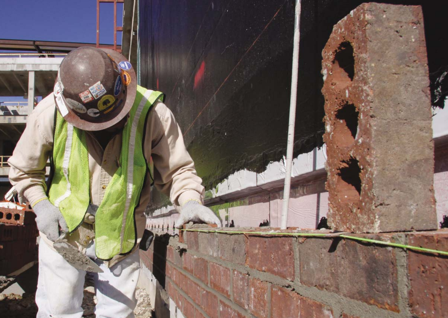
R.O.C. Construction and Masonry aligns bricks on the southwest corner of the east wing of the second UNT Dallas building in January 2010.
