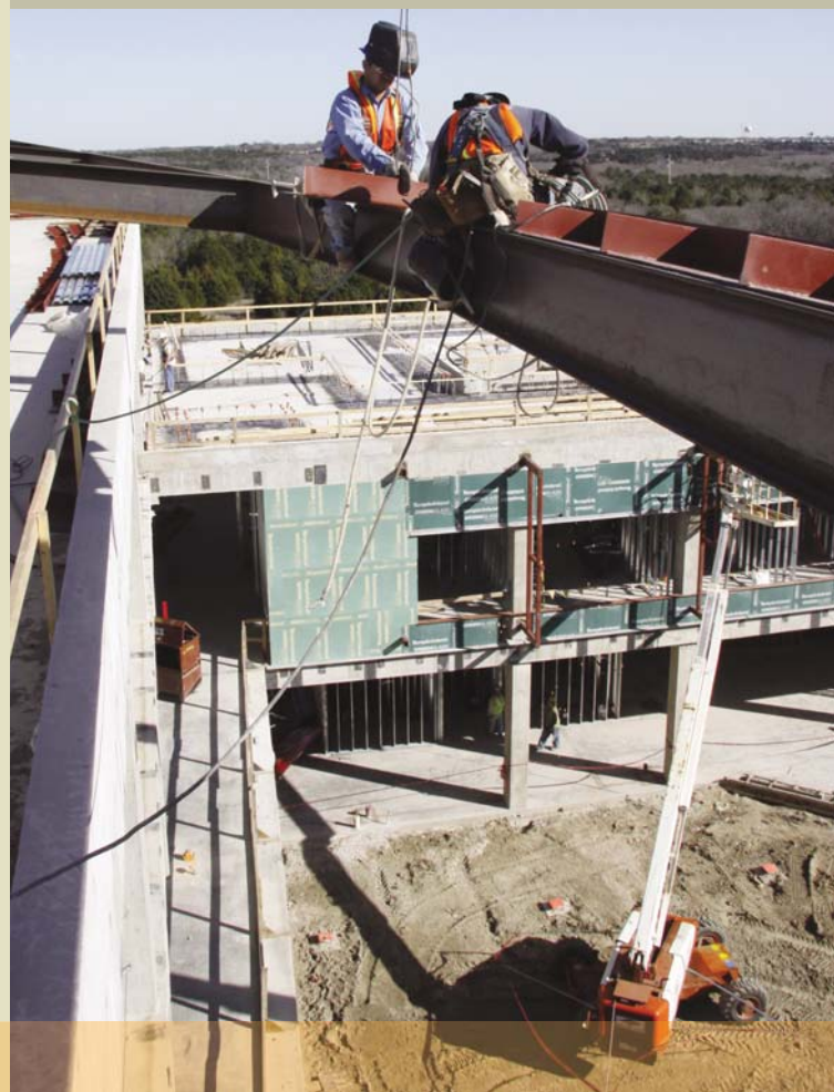
Members of Beck Construction weld pieces of steel to the roof marking the edge of the building.
